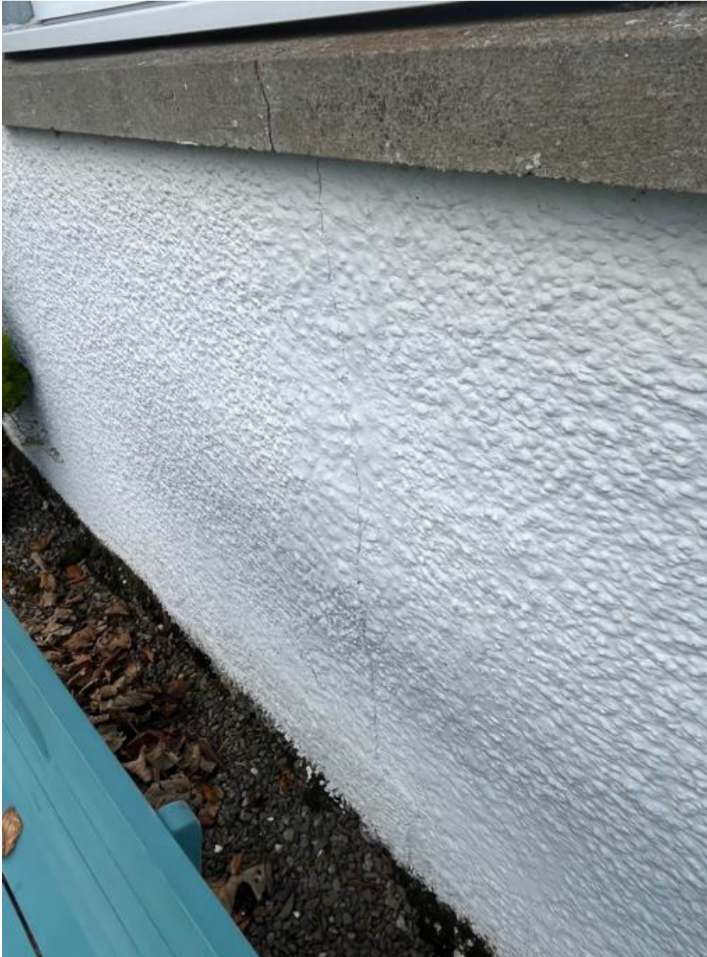
Photo 1 - Crack below window
