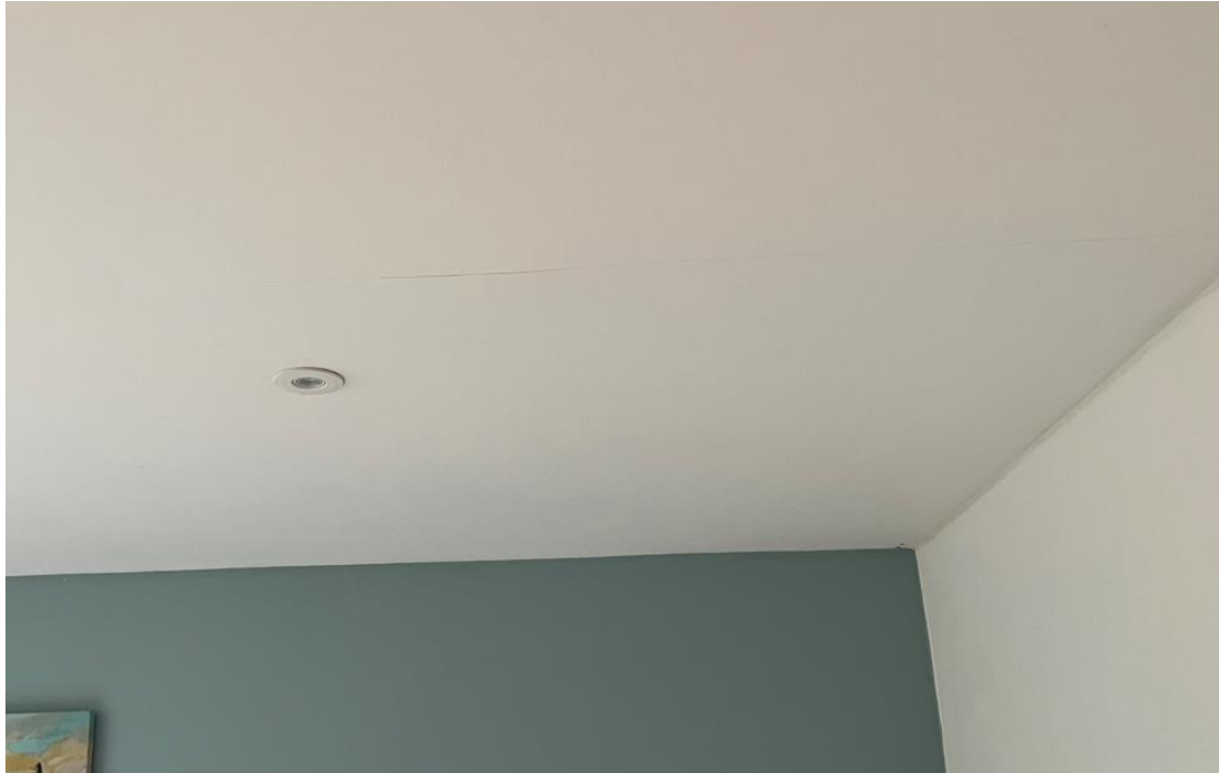
Photo 2 - Crack in ceiling
