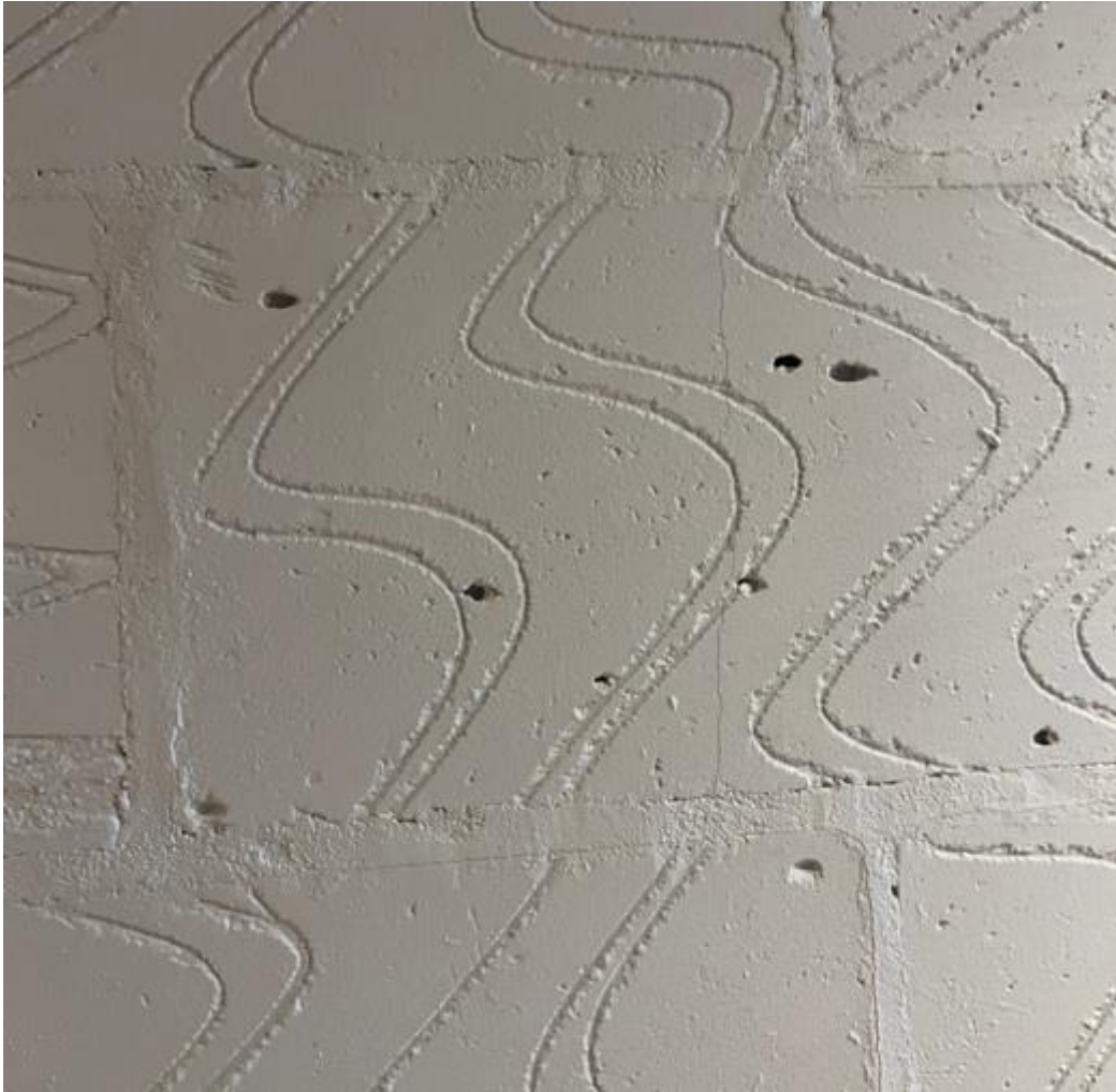
Photo 5 - Cracks in hall / bathroom wall
