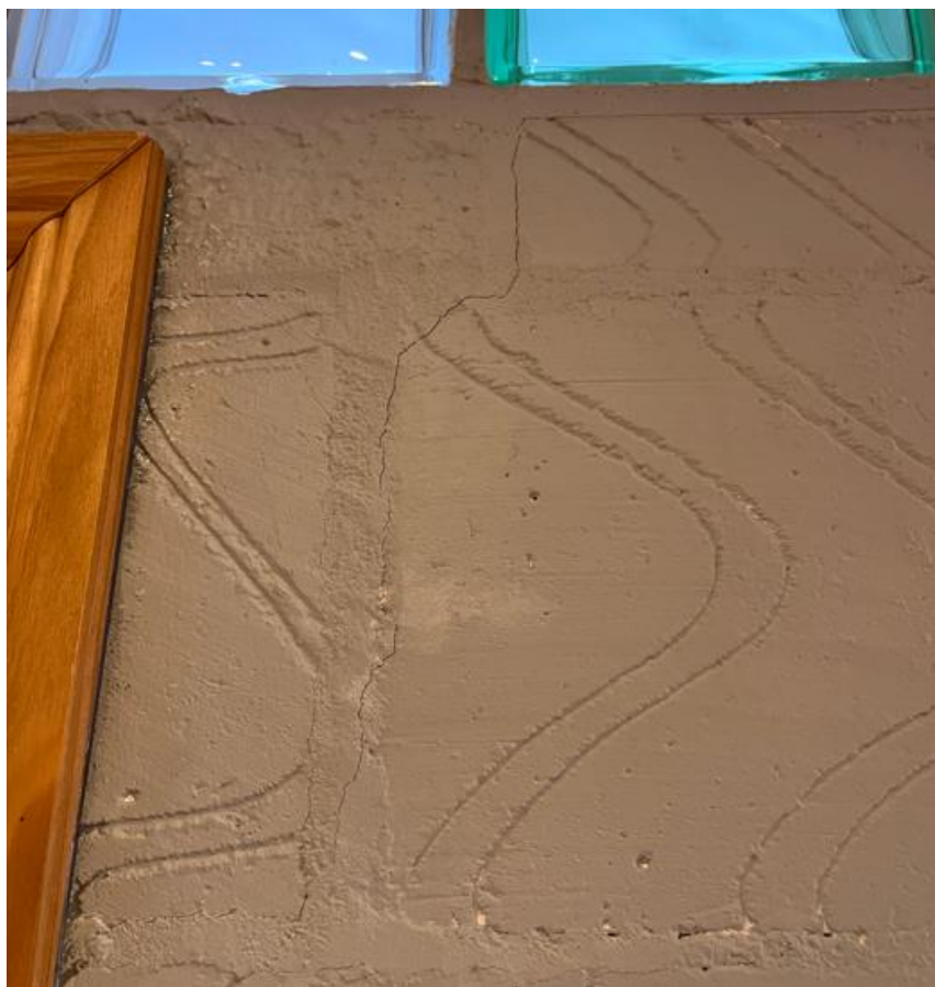
Photo 3 - Cracks in hall / bathroom wall
