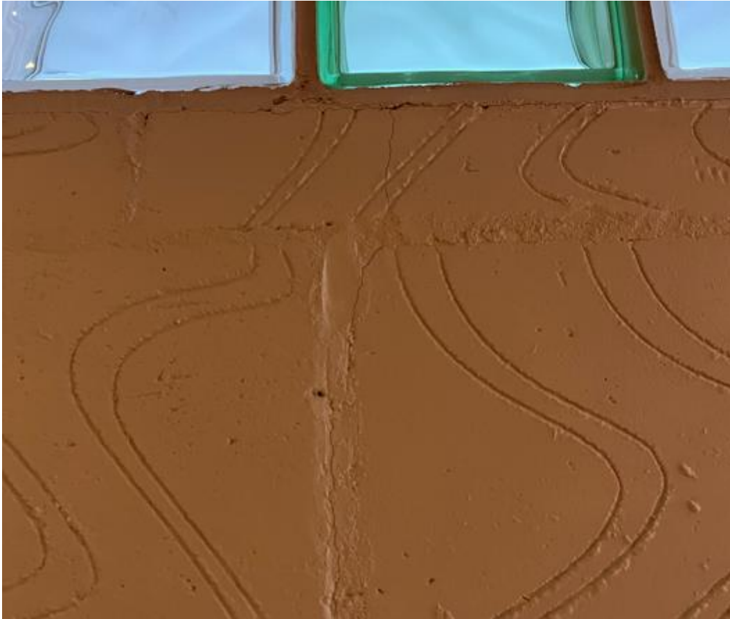
Photo 4 - Cracks in hall / bathroom wall
